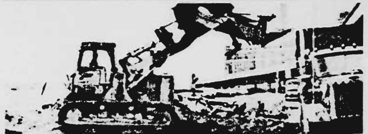
BULLDOZERS AWAY: Workers clearing rubble from the former home of the Transit-Mix cement company on the East River at 20th Street. The company has been ordered to restore the site to its original condition and the N.Y.C. Department of Ports and Terminals reports that "work is going smoothly."
